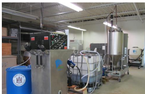
This is the system currently being used to covert waste vegetable oils to biodiesel at the AAMU CALNS greenhouse.
